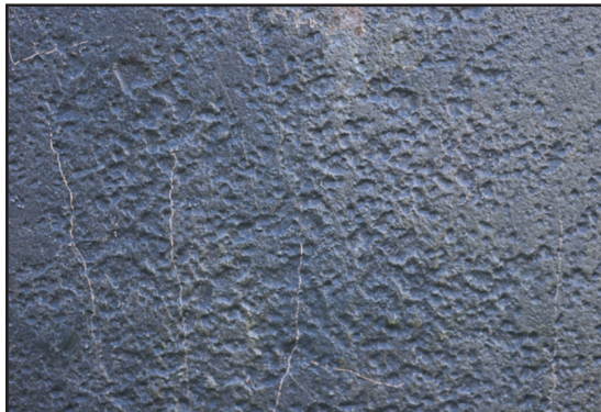
Pitting corrosion on structural steel
